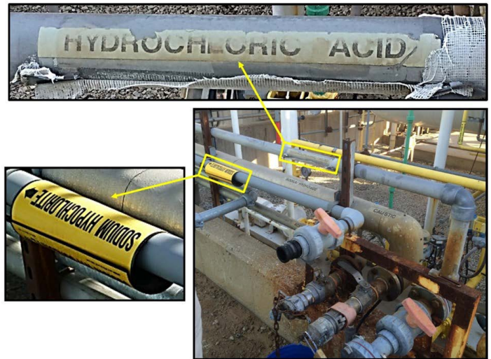
Figure 12. Sodium hypochlorite pipe marker appearing upside down (left) and sulfuric acid piping mislabeled “hydrochloric acid” from a prior service (top). Both pipe markers are located several feet from the fill line and elbow (right) (Source: CSB).
