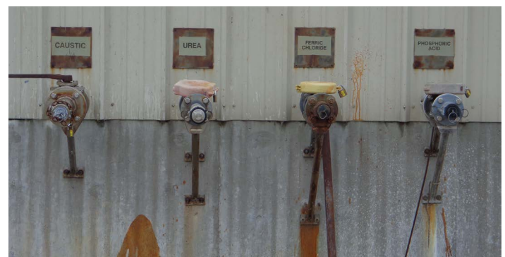
Figure 13. WWTP chemical fill lines (Source: CSB).
